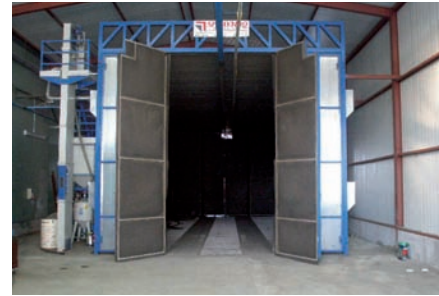
Sala de granalla Metallic grit blasting room
